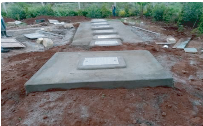
Completed water treatment system
